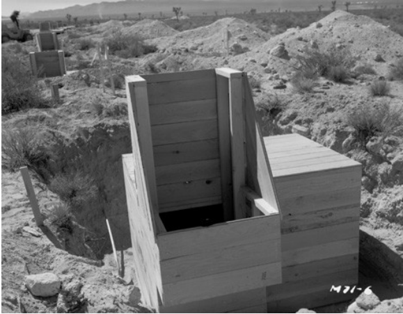
Personal Shelters, BUSTER {9.1a}, about 6 ft on a side, before being placed underground
